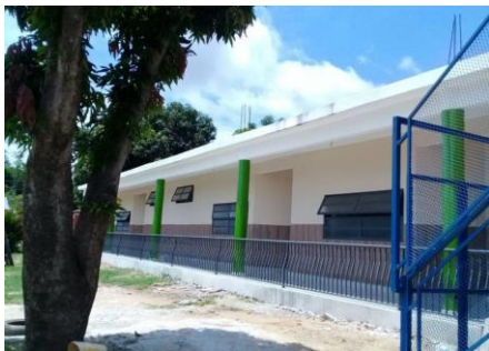
2017 original school demolished and a greatly enlarged new school built to meet increased need.
